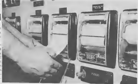
ROUGHPUT is continuously and accurately recorded on delicate flow recorder control instruments installed in unit control houses.
